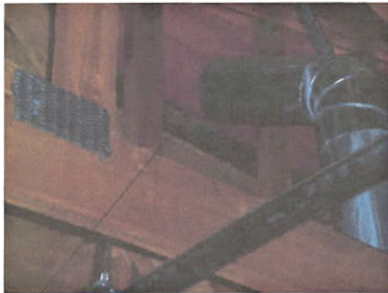
Photograph #2 HVAC Heater Vents Not Exhausted Directly to Outside
