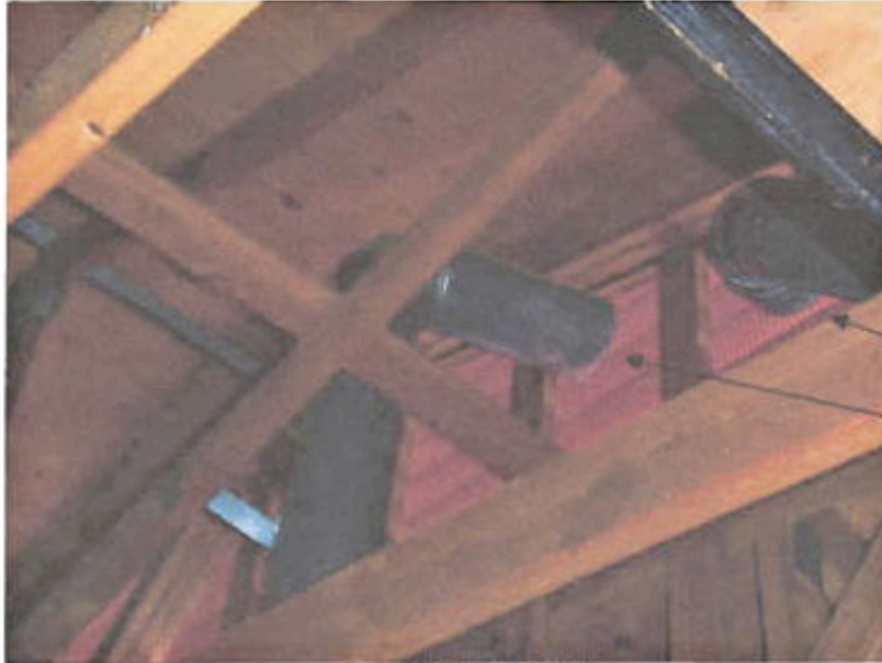
Photograph #1 HVAC Heater Vents Not Exhausted Directly to Outside
