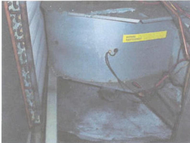
Photograph #4 HVAC Condensate Pan Residue
