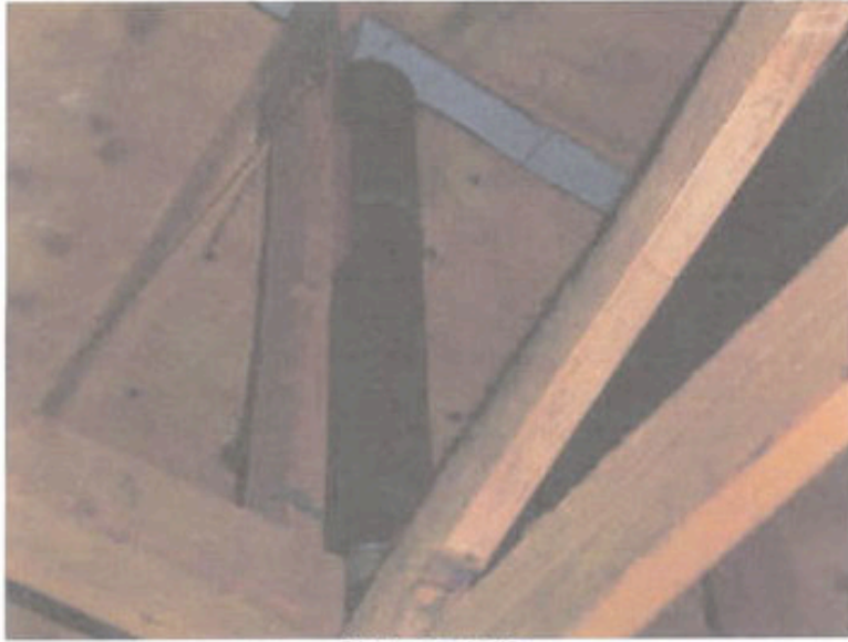
Photograph #3 Sanitary Vent Not Exhausted Directly to Outside
