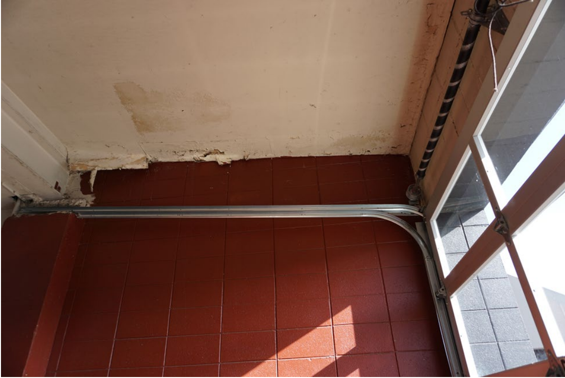
Leaking Roof Ceiling on North Side of Station 50
