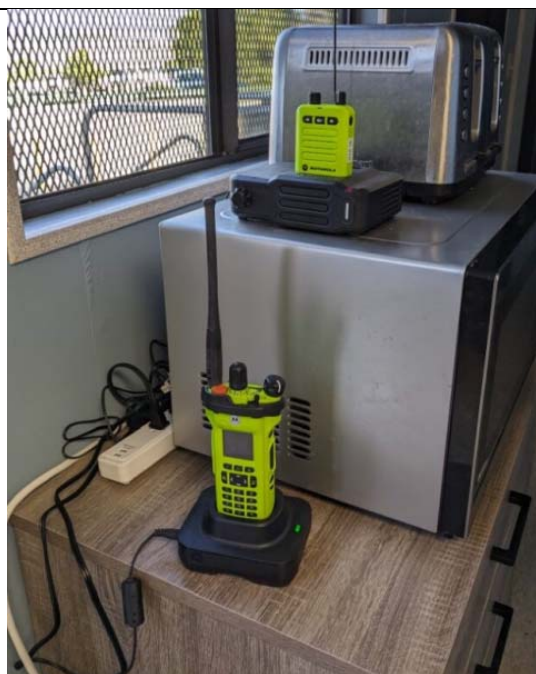
Alert system in modular trailer
