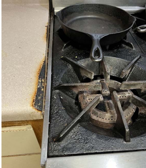
Old stove/countertop damage
