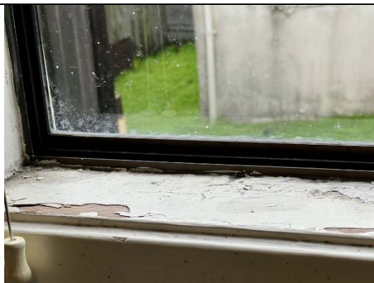
Window sill paint peeling
