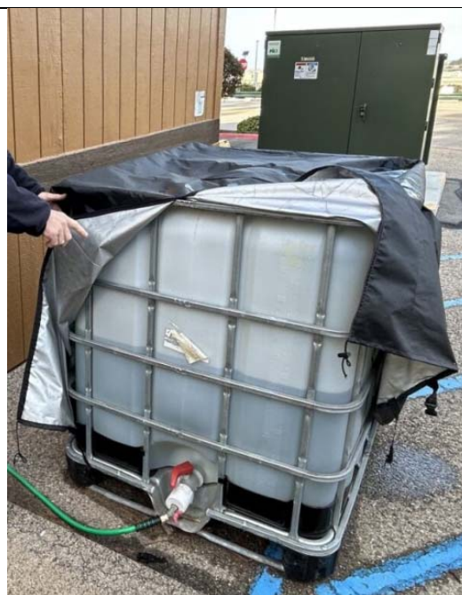
Non-potable water supply
