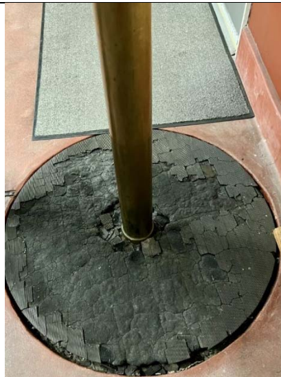
Poor condition of fire pole landing pad
