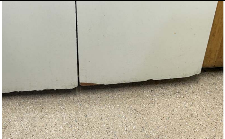
Chipped/worn out kitchen cabinetry
