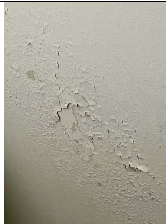
Kitchen paint flaking/peeling
