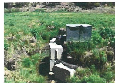
Steam-bed erosion jeopardizes pump # 2
