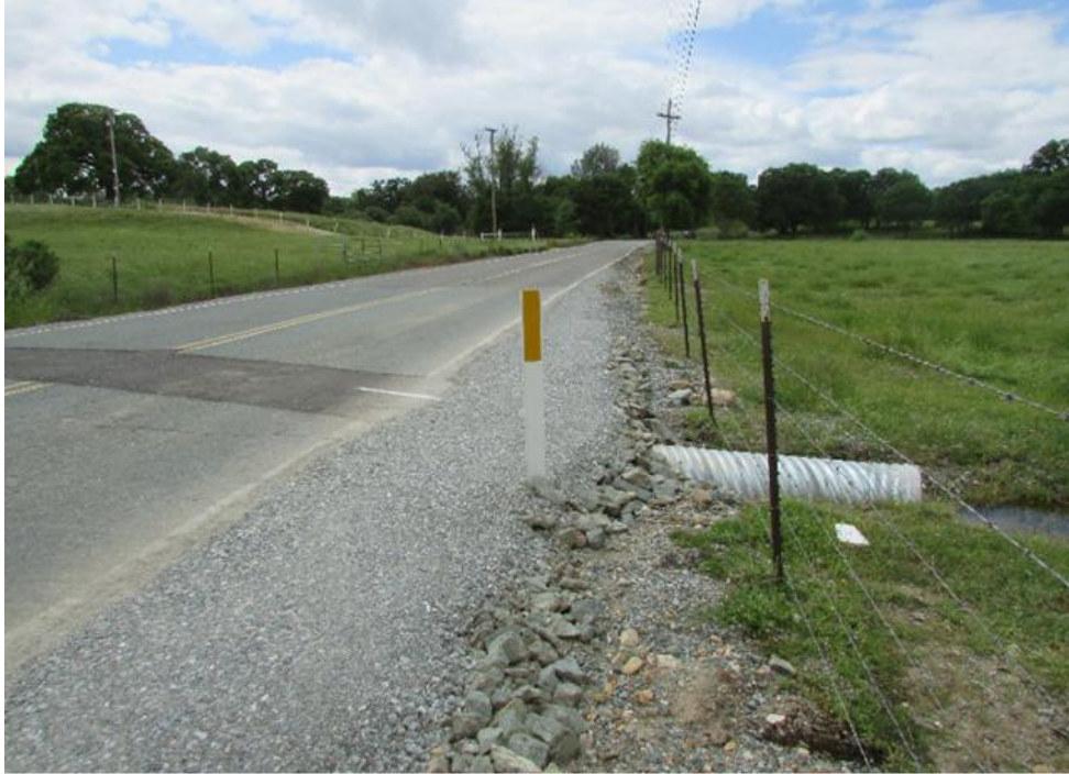
The eastern end of the .4 mile section with 16-18 transitions of section-replaced pavement. The culvert in this view is the recently replaced 18” one mentioned above.
