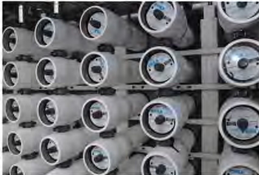
Bank of Desalination Membrane Filtering Tubes
