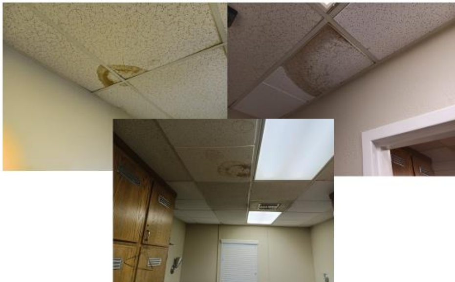
Photos provided by the Grand Jury (Station 45 water damaged ceiling tiles)
