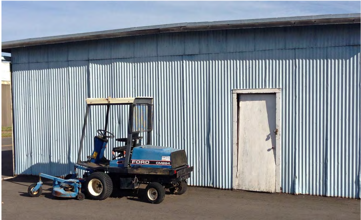
Figure 5. This equipment is stored out in the weather next to a hangar that needs serious maintenance along with paint.
