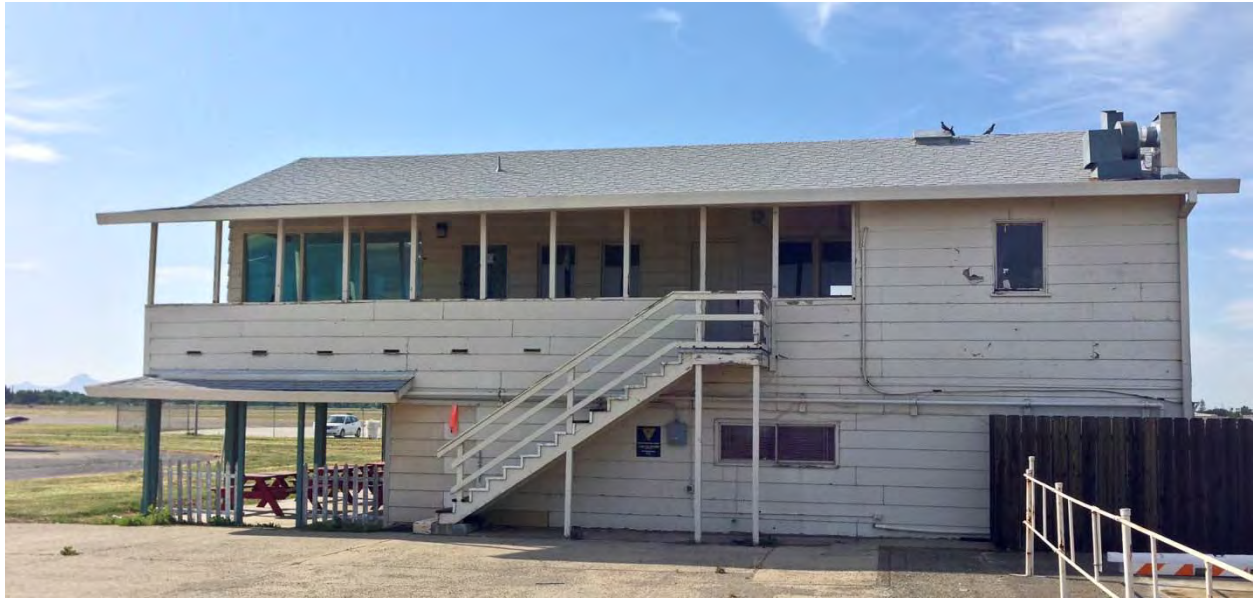
Figure 4. This airport building is in need of paint and maintenance. Airport buildings do not have scheduled maintenance and are now showing signs of wear. The exposed wood and leaking roofs are beginning to require funding and maintenance. Aircraft and equipment are reportedly getting wet in these facilities because of leaking roofs.
