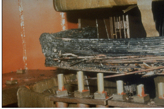
Salem New Jersey transformer at nuclear plant damage from solar flare, 1989 41 Salem New Jersey is at 39.58 North Latitude
