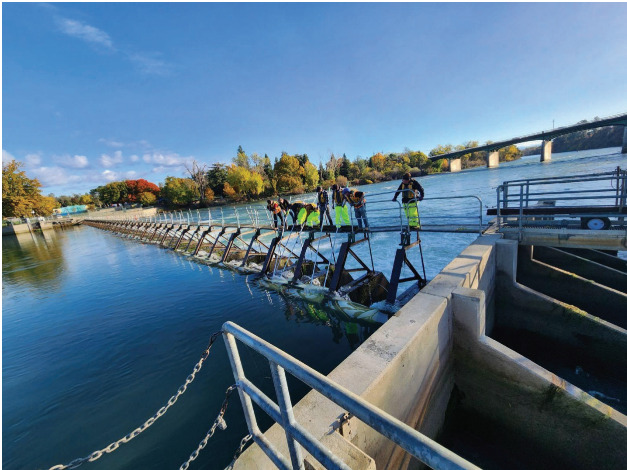
ACID employees erecting the diversion dam for another irrigation season. Photo used with permission by ACID Board of Directors.
