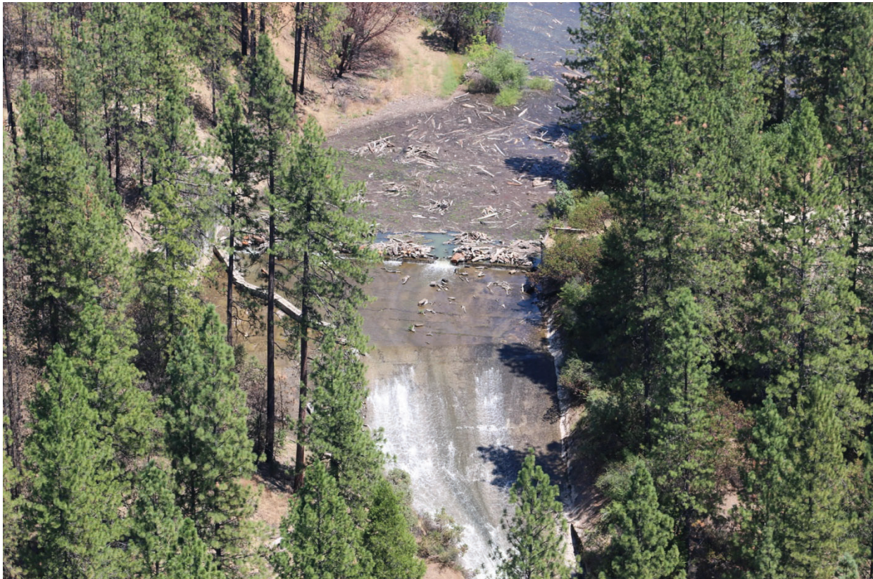
Water and debris flowing over the Misselbeck Dam Spillway. Photo by permission of Igo-Ono Community Services District.
