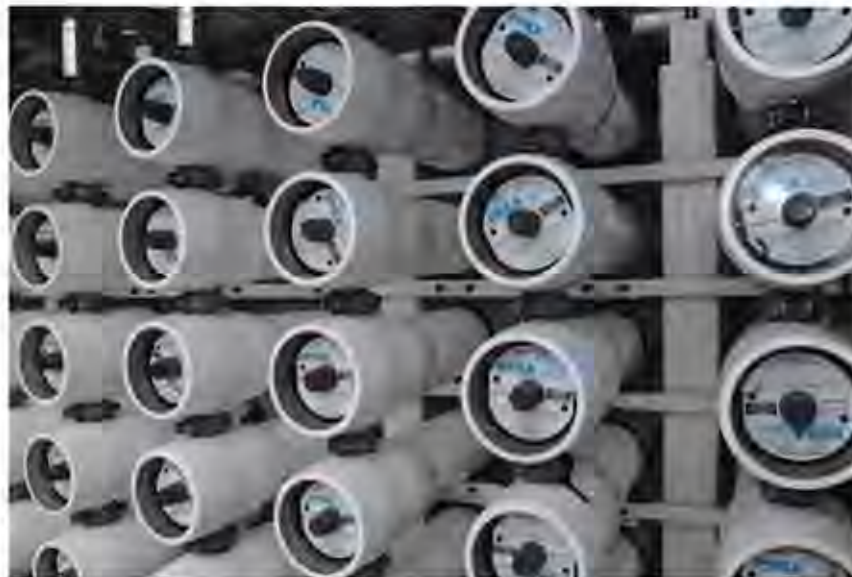
Bank of Desalination Membrane Filtering Tubes
