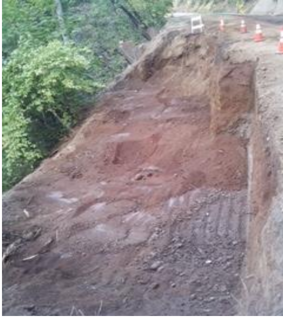
One damaged section of Shake Ridge Road, Fall 2017
