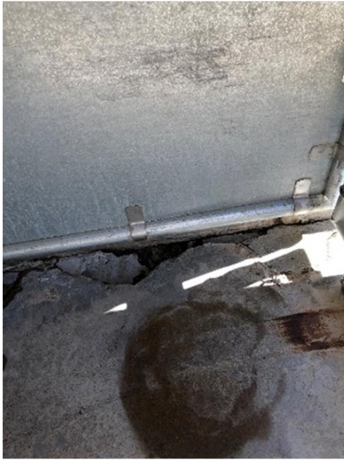
Fig. 3 - Crack in floor/wall - dog kennel area
