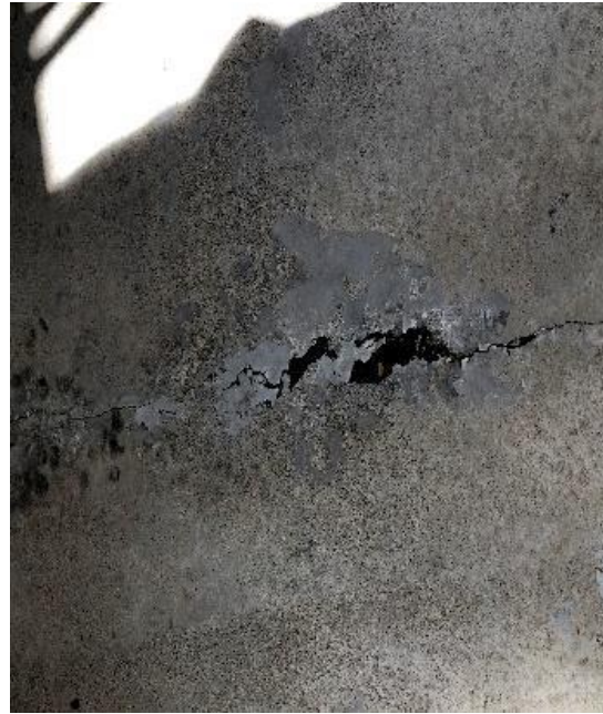
Fig. 4 - Hole and crack in dog kennel floor
