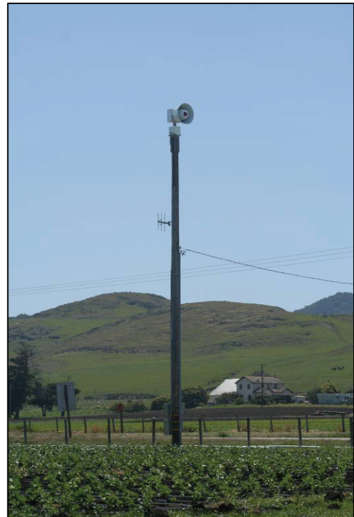
Emergency Alert Siren – Photo by Brandt Kehoe
