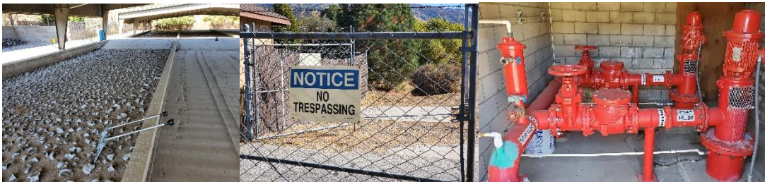
(Photos by the Grand Jury showing Water Reclamation Plant, October 10, 2019)
