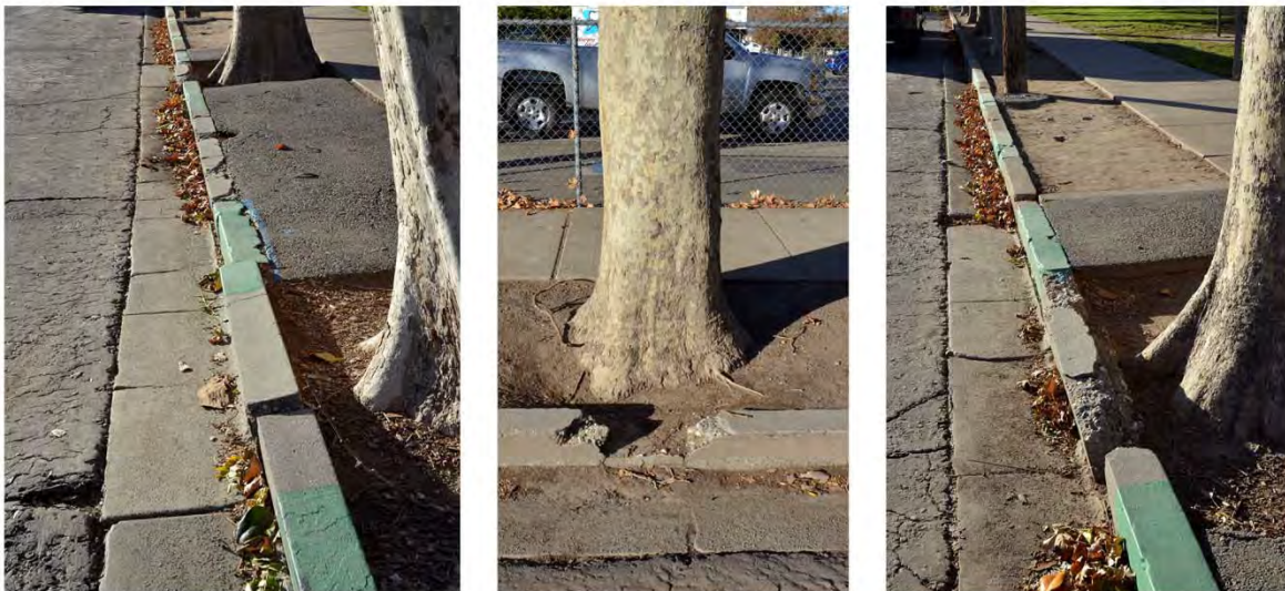
Figure 3. Broken Curbs on the part of 7 th Street that traverses the Covillaud Elementary campus.
