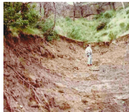
Photo 1: Landslide caused by break in pipeline, January 1980 Photo provided by Amador Water Agency
